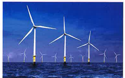
▲ Wind turbines in the sea
